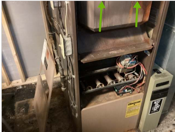
Rusted chamber with holes in flue
