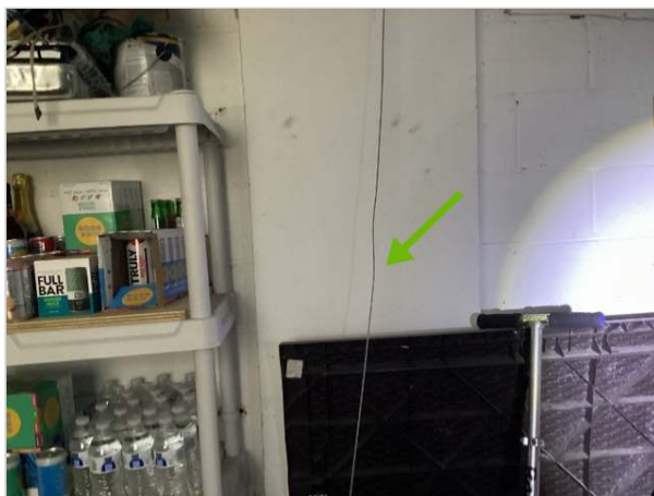
Right cable loose
